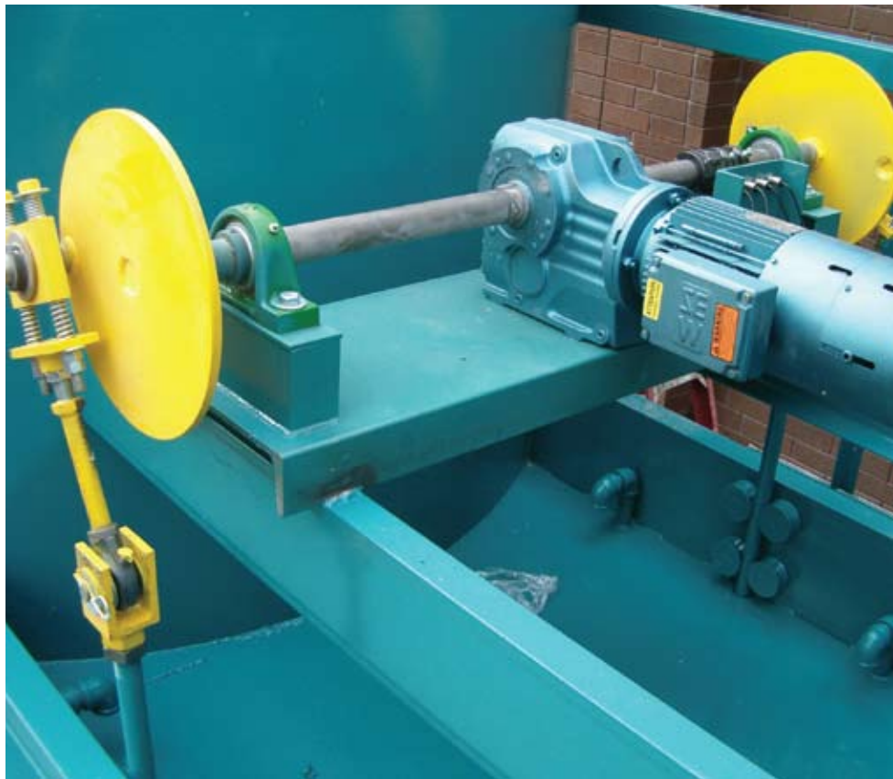
Above is an example of an electrically controlled valve system. Maintenance time and expense is greatly reduced.
